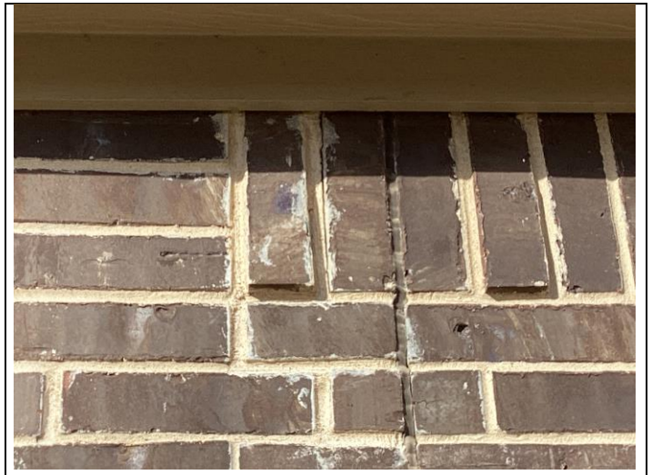
Sample of brickwork/mortar cracks
