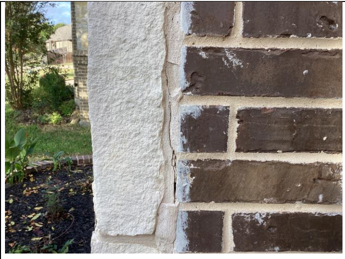
Sample of stonework/mortar cracks
