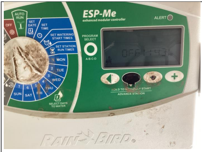
Photo of damaged/missing button
