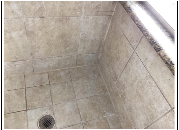
Sample of deteriorated grout
