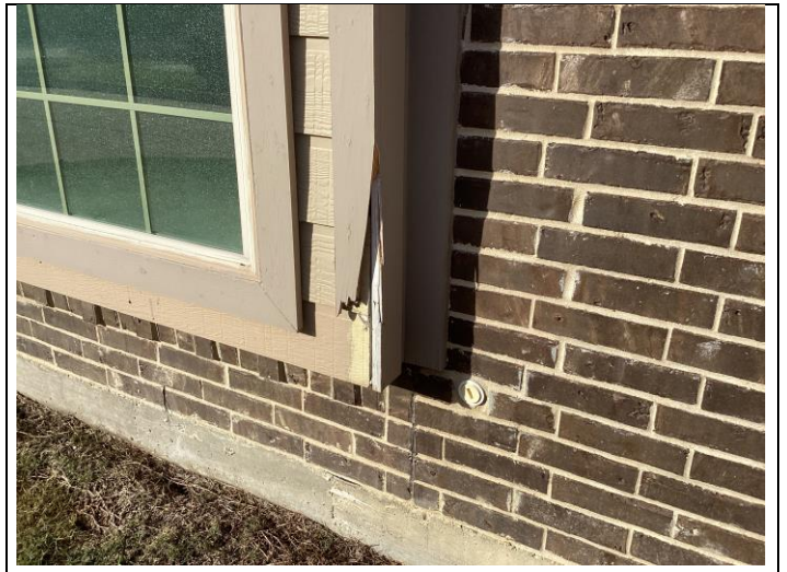
Sample of damaged trim
