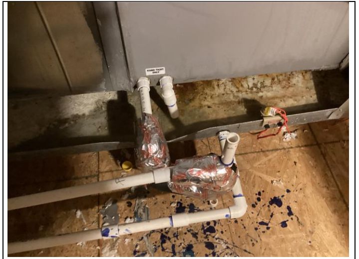
Photo of water collecting in the A/C drain pan
