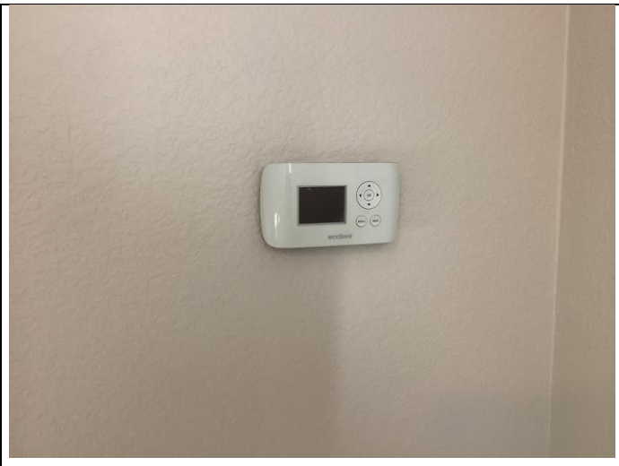
Photo of inoperative A/C thermostat
