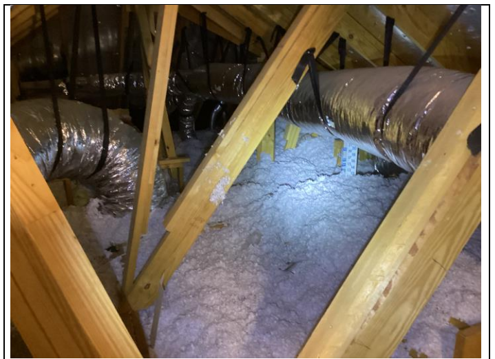
Sample of indication of tunnelling/compressed insulation
