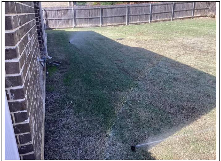
Sample of sprinkler system operating
