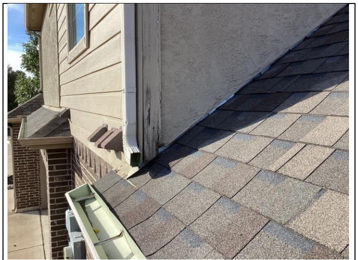
Sample of deteriorated/damaged trim
