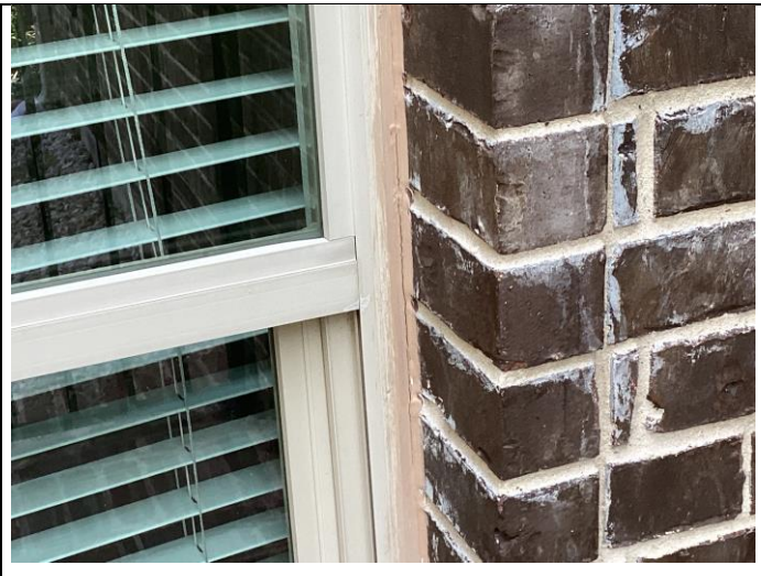
Sample of gapped window caulking/missing screens
