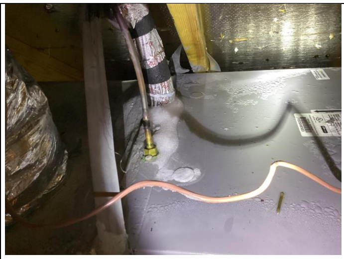
Photo of iced A/C coils/suction lines
