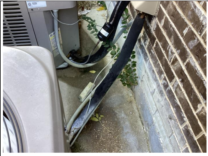
Sample of deteriorated A/C suction line insulation
